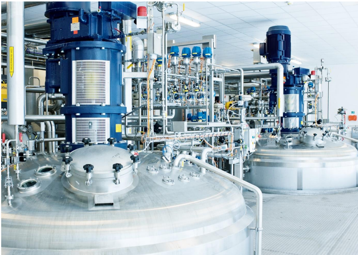
Figure 1 - Batch Reactor Train
